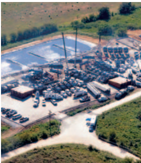
BJ's "simo-frac" technique has proved successful in horizontal wells in shale reservoirs. Here BJ crews frac three horizontal shale gas wells at once.
