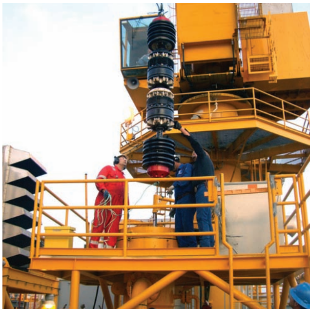
Fig. 3—TDW Offshore's SmartPlug high-pressure-pipeline isolation tool being delivered to the Enterprise Independence Hub platform.
