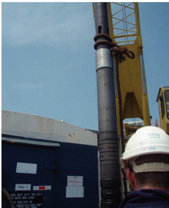
Fig. 2—An RBP with an MTM seal is shown during installation in the BKC-20 well at the Bunga Kekwa field in Malaysia.
