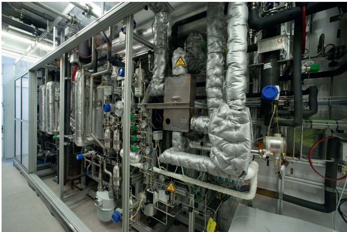
Fig. 2—FT section of the UK pilot plant.
