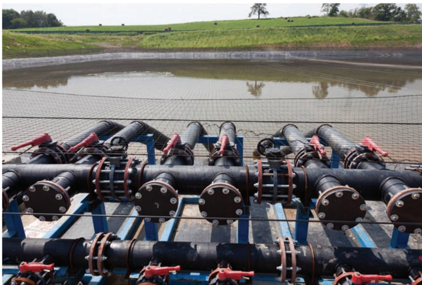
These pipes connect a treatment pond to well sites where water produced from nearby shale gas wells is reused for fracturing. Netting keeps out birds and two liners plus an alarm system are used to prevent leaks.
