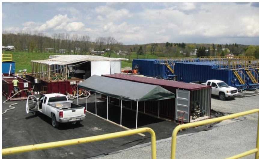
This portable water treatment system is able to process 10,000 b/d of produced water for reuse in fracturing gas wells in the Marcellus Shale in Pennsylvania. The series of units remove minerals, clarifies the water and reduces the volume of the solids that can reduce a field’s output.
